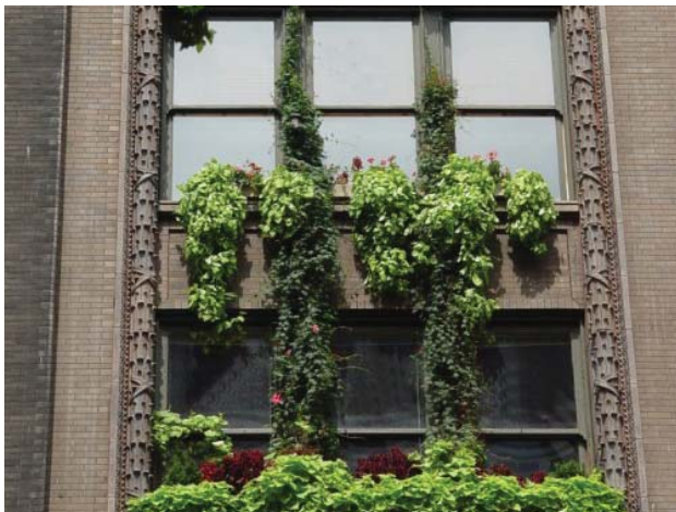
Seasonal plantings comprised of Carolinian plant materials enhance the visual interest of this façade
